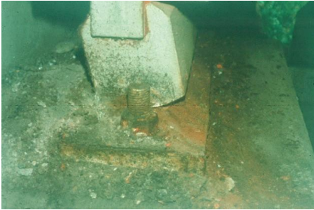
Segmental rocker bearing (out of position)
