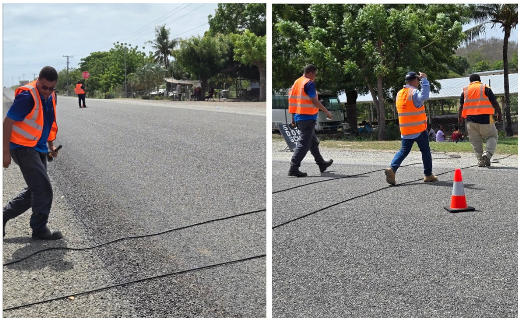
Typical example of setting out details of MetroCount device during installation and uninstallation. Note Dayglow vests, STOP/SLOW signs and road cones to help manage safety on site
